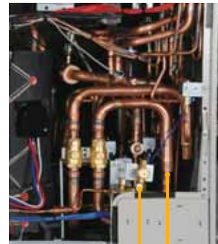
Liquid pipe Gas pipe
